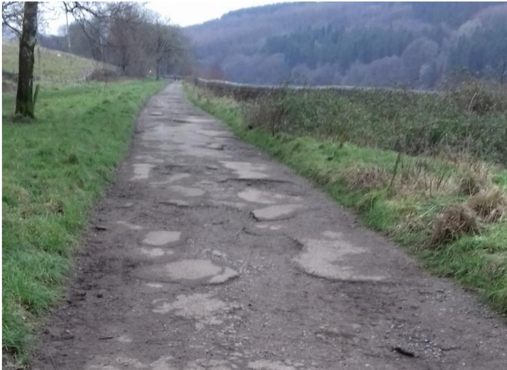
Figure 3. The potholed, uneven approach road
